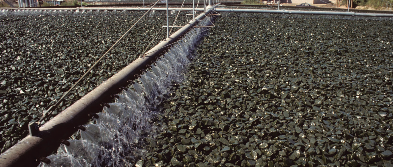
Wastewater Treatment Plant in Danbury, Connecticut. UN Photo/Evan Schneide
